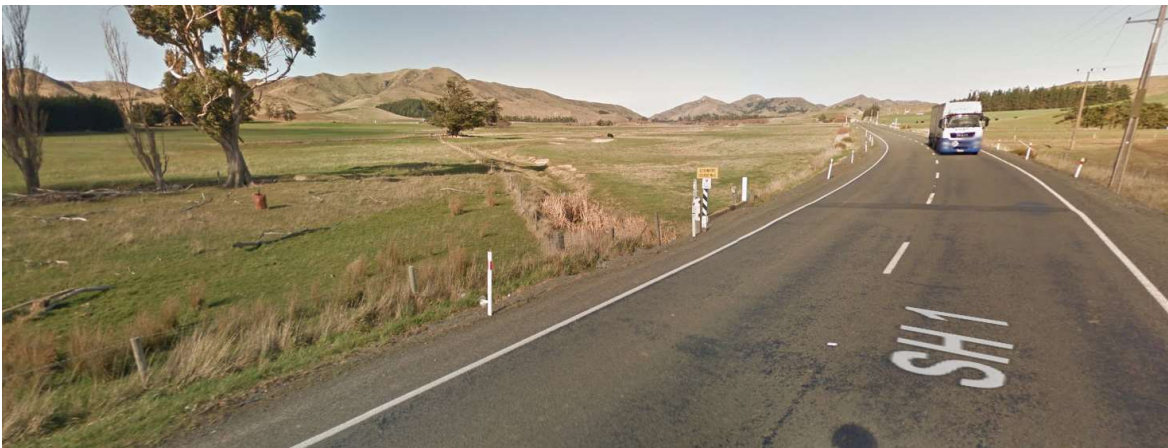
Figure 4-1: Example of drainage culvert under the SH1 taken from Google maps near Taimate.
